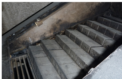
wood chip furnace – mobile grate
