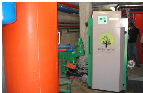
wood boiler and heat storage
